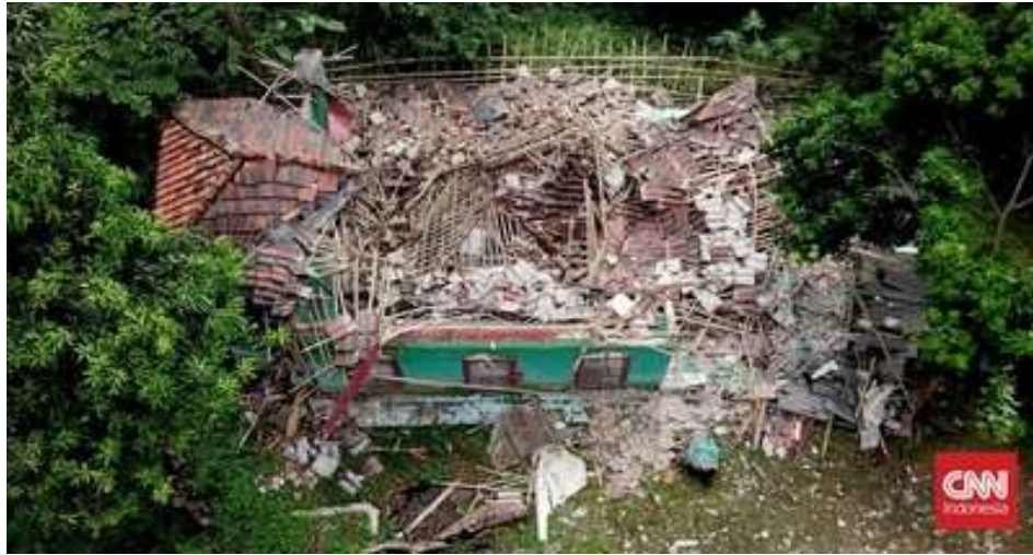
Figure 1. Damaged Building (Source: CNN Indonesia)
